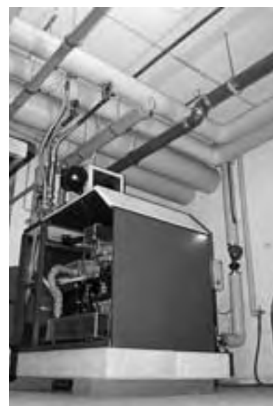
Decentral CHP plant
