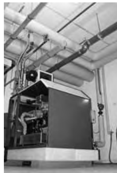
Decentral CHP plant
